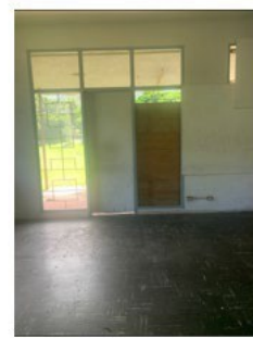
Windows and Doors Need Repair
