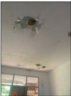
Extensive Ceiling Damage Throughout the Inside
