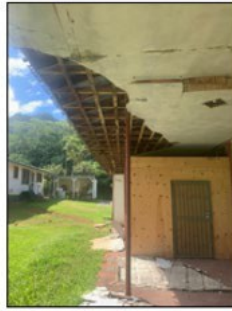
Patio Wall has Collapsed and Ceiling Has Fallen
