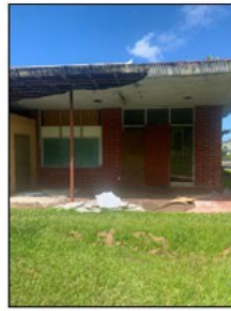
Ceiling Damage and Old Boards to Cover Windows
